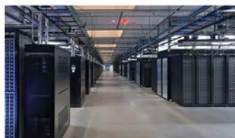
HOT AISLE CONTAINMENT
