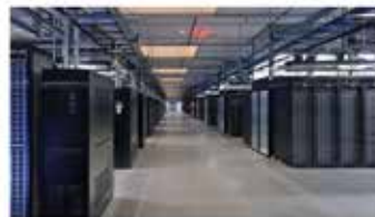
HOT AISLE CONTAINMENT
