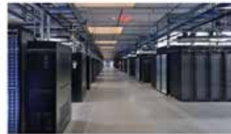
HOT AISLE CONTAINMENT
